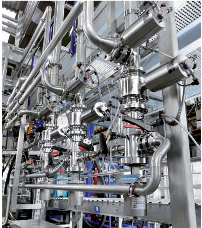
KIESELMANN pigging system in a production plant
